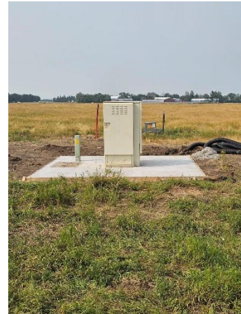
(Above) A newly installed fiber distribution cabinet serves as a key network hub supporting West River's completed broadband expansion project.
